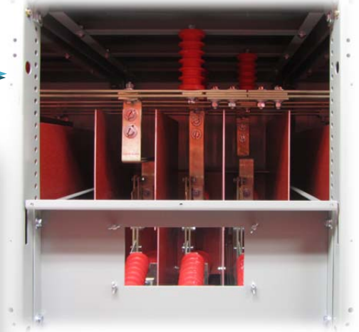
Figure 4: Main Bus with Visual Disconnect Window Removed
