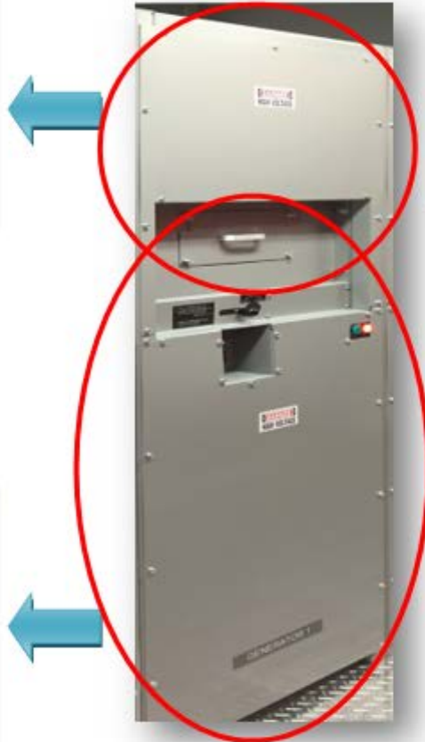
Figure 2: Single Front Access Section with Dead Fronts Attached
