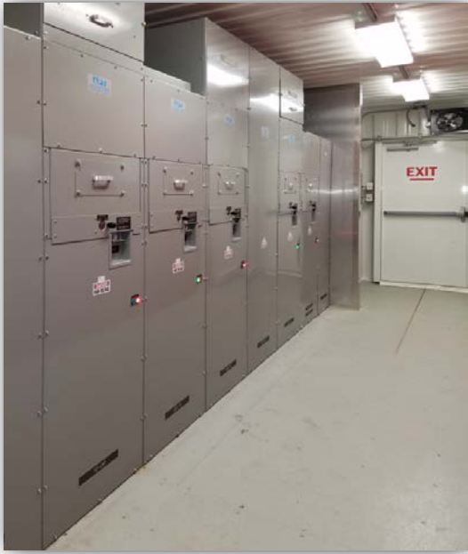
Figure 1: Modified 40' container down to 30' Mobile Container-Based Walk-in Switchgear
