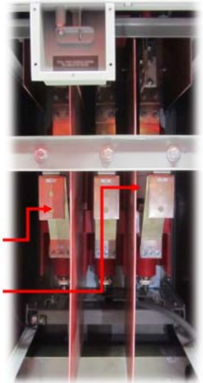
Figure 6: Inside cable connection compartment
