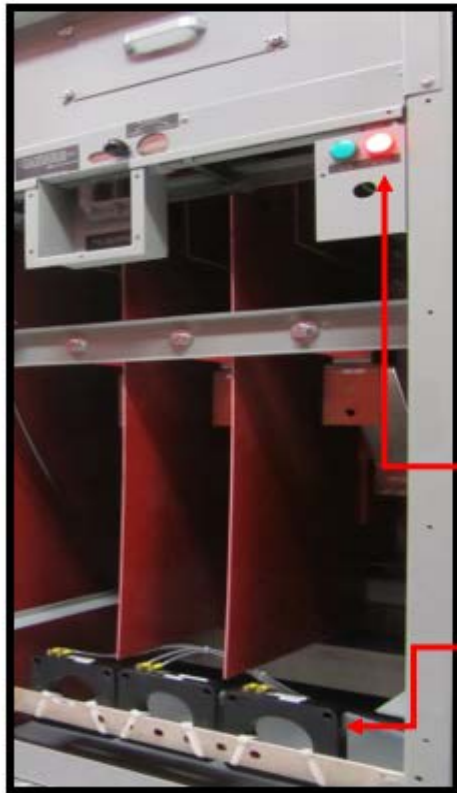
Figure 5: Cable Connection Compartment Dead Front Removed
