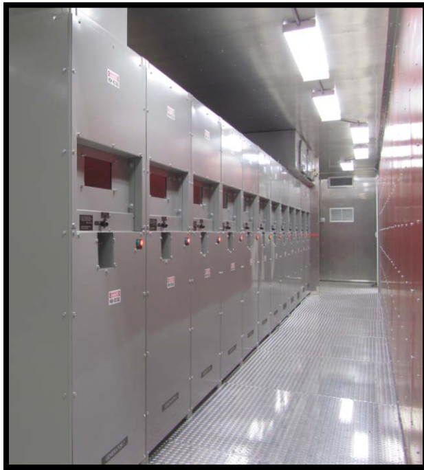
Figure 8: Inside of ISO Container based Switchgear Module with Ultra Compact Front Access (FA) Air Insulated Vacuum Circuit Breaker Switchgear
