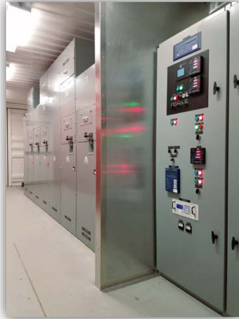
Figure 2: Interior of Mobile Container-Based Walk-in Switchgear including Isolated Master Control Panel
