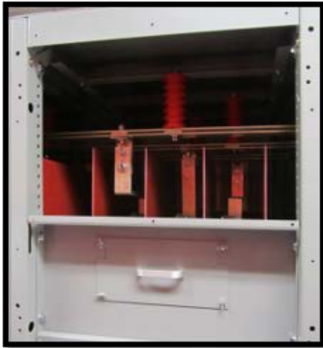
Figure 3: Dead Front Removed Exposing Main Bus Compartment with Cover Over Visual Disconnect Window
