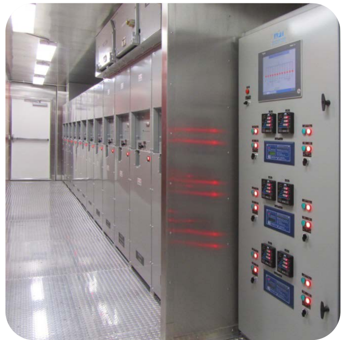
Figure 7: Front Access Switchgear, Isolated from Local and Remote Operator Control Stations
