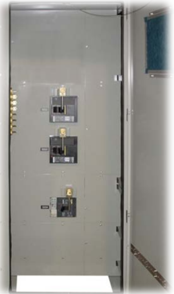
Figure 8: Auxiliary Feeder Section w/ Kirk Key Transfer Block & Interlocks*
